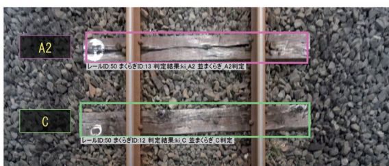
Fig. 9 Detection of wooden sleepers and deterioration evaluation results
