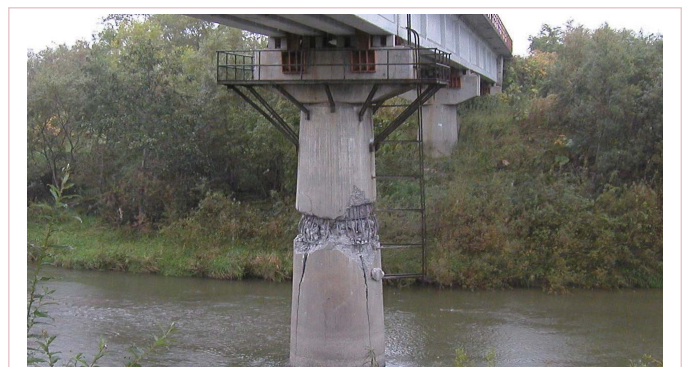
▶ Example of damaged section containing termination of longitudinal bars in bridge pier
