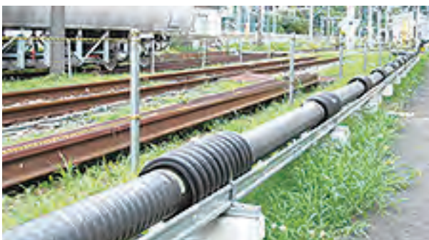
Figure 4-8-1 Installed 300-m class superconducting feeding feeder cable
