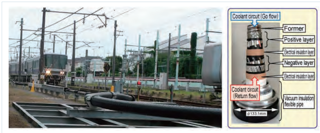
fig.1 310 m superconducting feeder cable
