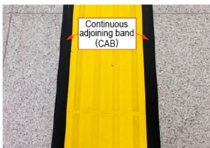
Fig.3 Example of continuous adjoining bands (CABs) with TWSIs
