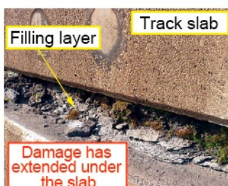
Fig 3 Example of extensive deterioration (condition at the surface)
