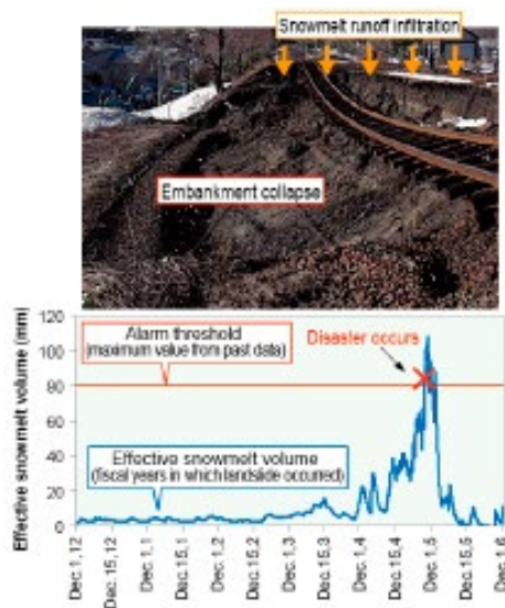
Fig.1 An example of an inspection of an earth-bank slope in critical condition.
