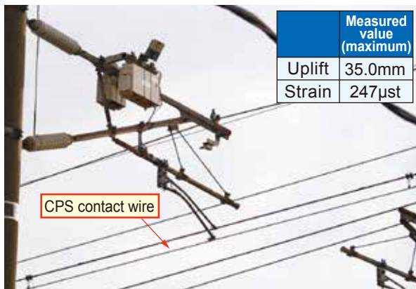
Fig.3 Image of test installation of CPS contact wire on a Shinkansen line and results of dynamic characteristic measurements
