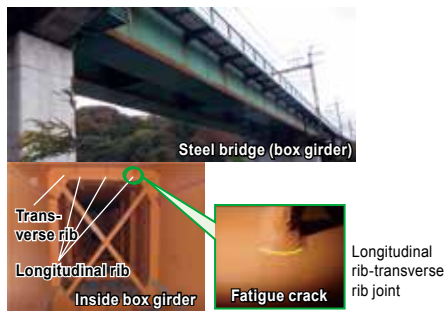
Fig. 1 Fatigue cracks in the vicinity of rail joints
