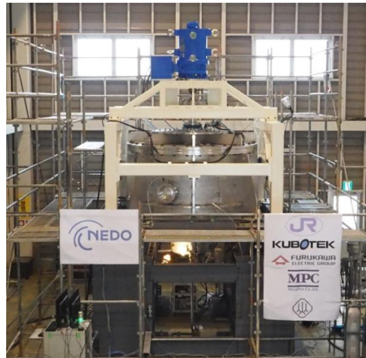
The superconducting flywheel power storage system
