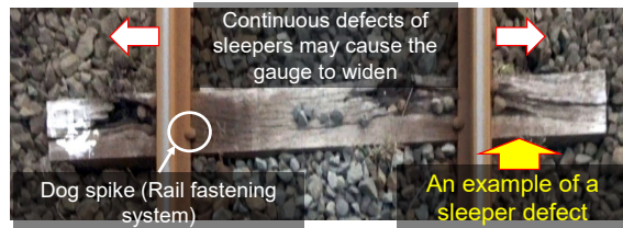
Fig. 2 An example of a sleeper defect
