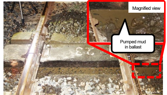
Reference photo Fouled ballast
