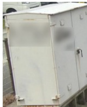
Fig. 11 Least deteriorated level crossing equipment box
