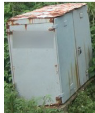
Fig. 10 Most deteriorated level crossing equipment box
