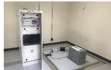
Earthquake early warning system
